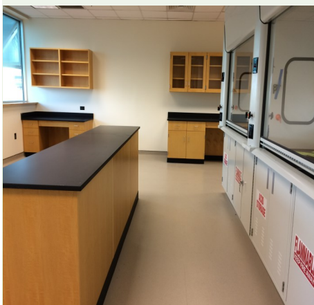
NCF 273—NCF Organic Chemistry Research Lab Fume Hoods
